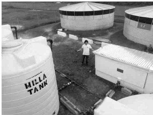
Photograph 1. Water tanks area
